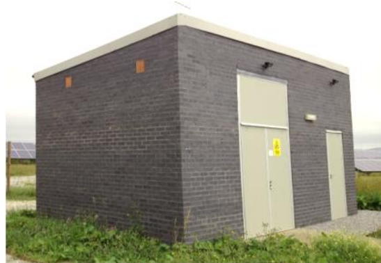
DNO Substation, Little Trevease Cornwall
