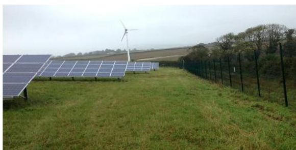
Ninnis Solar Farm, Cornwall
