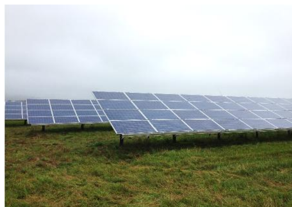
Ninnis Solar Farm, Cornwall
