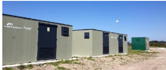
Inverter (centre), Little Trevease Solar Farm, Cornwall
