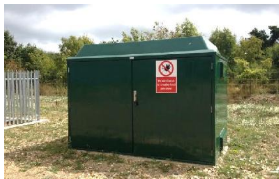
Customer Substation, Tavells Farm, Hampshire
