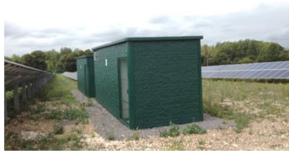
Inverter Building, Hatchlands Solar Farm, Devon
