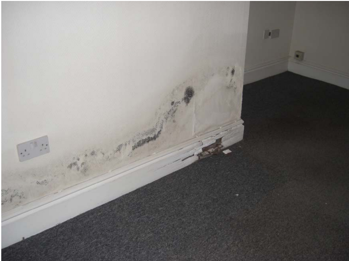
Damp to Office areas
