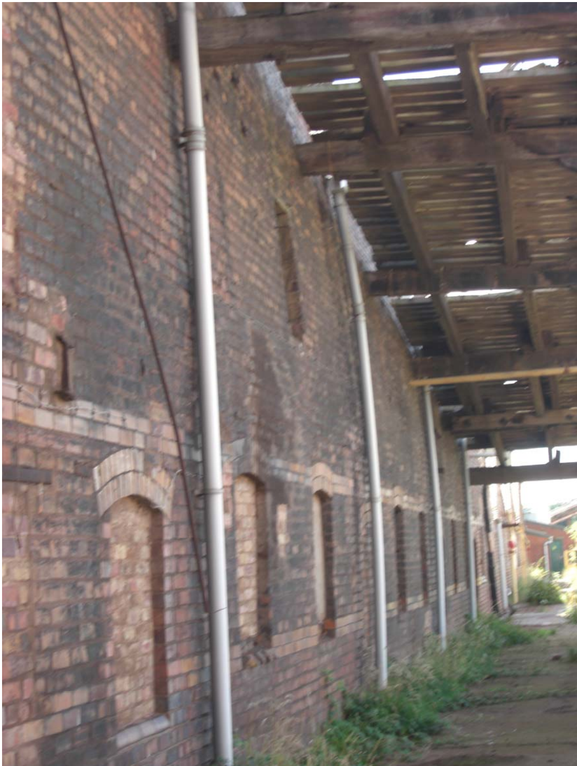
Rear of Part C Showing 'Lean In' of head to wall
