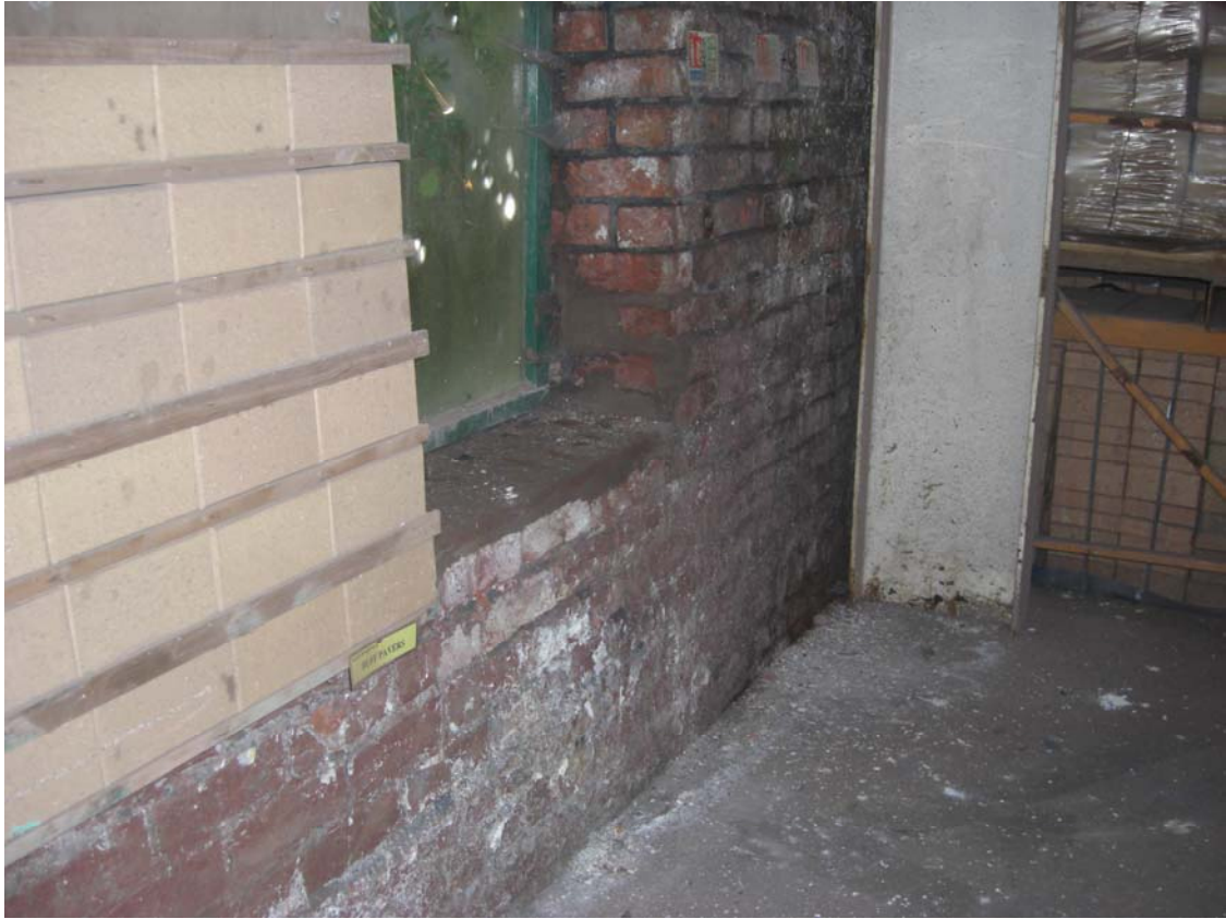
Typical low level damp Part A
