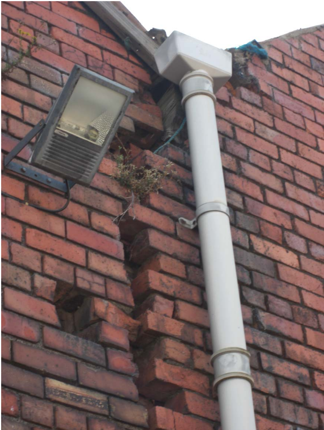
Rear Elevation Part B showing relative displacement at construction joint with Left Hand Side 'leaning in' at Head
