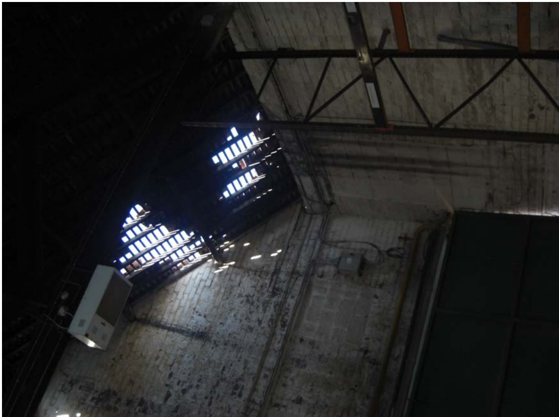
Typical Roof covering failure - Part B
