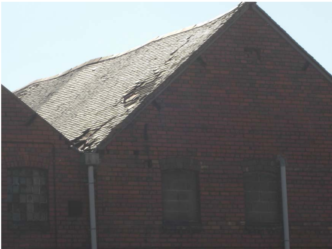
Deformed Roof & Damaged Tiling - Original Finish Part B
