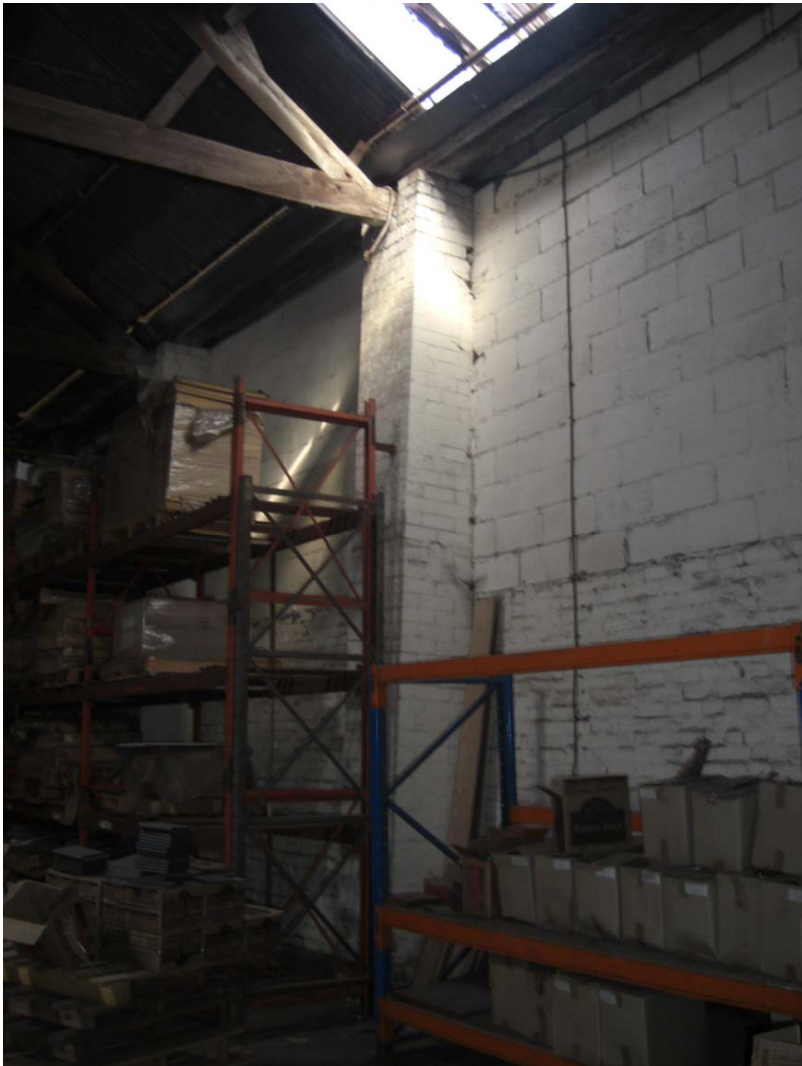
Out of Plumb wall / pier - Part B
