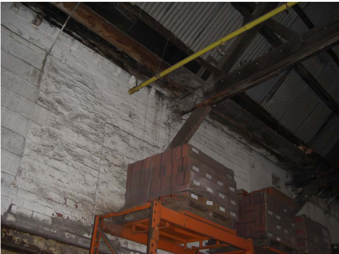
Water Penetration evidence at truss support / gutter - Part B
