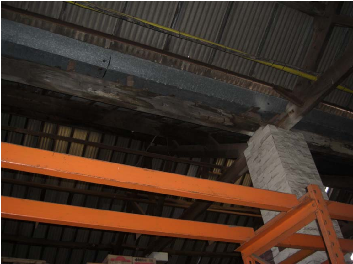
Replaced Internal Gutter with staining to timber support beam - Part B
