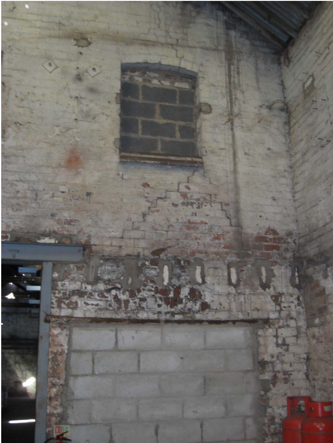
Typical Crack Damage to Part B
