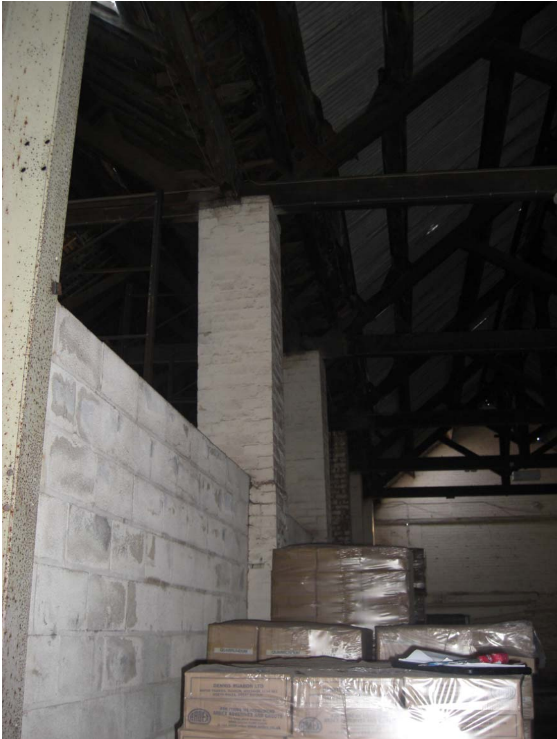
Out of plumb internal pier - Part B
