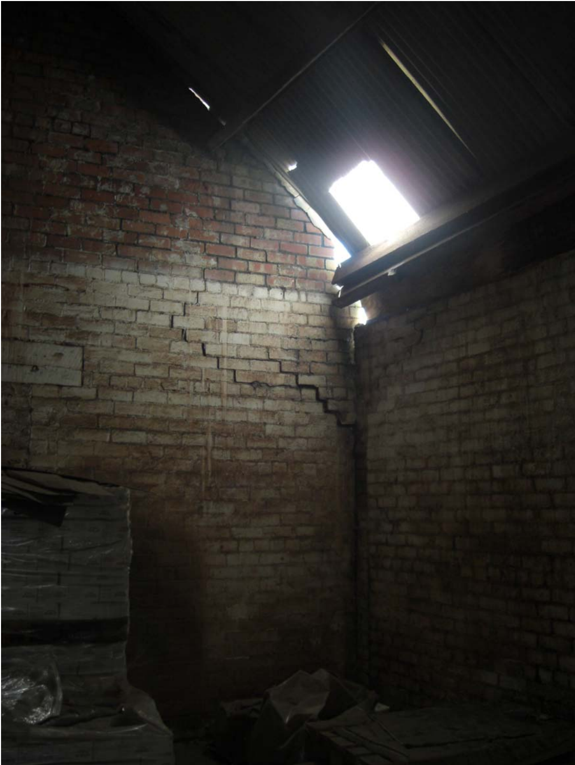
Internal with no support to timber beam
