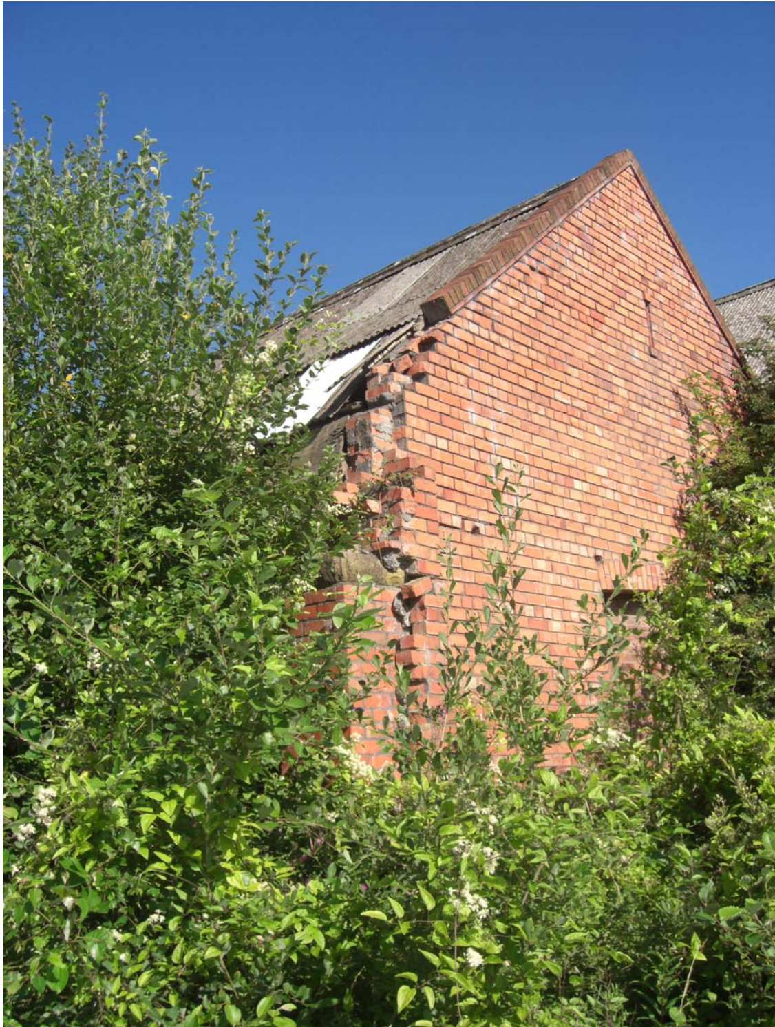
Damage to Front Part B Extension
