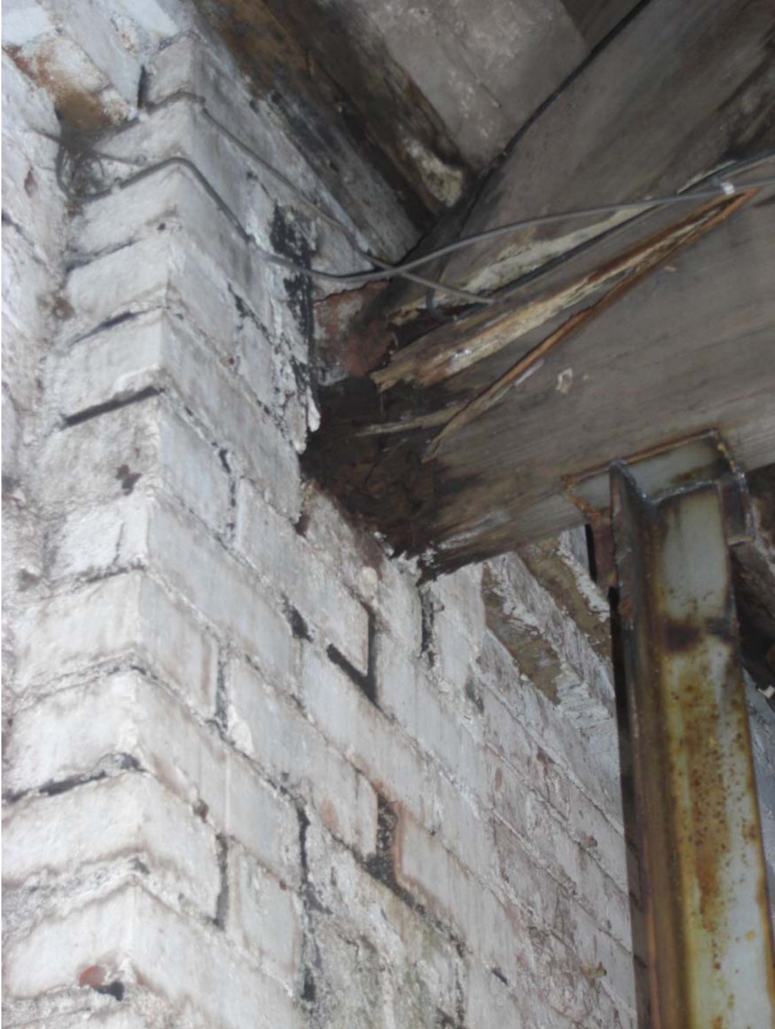
Failed truss support due to decay with steel prop – Part B
