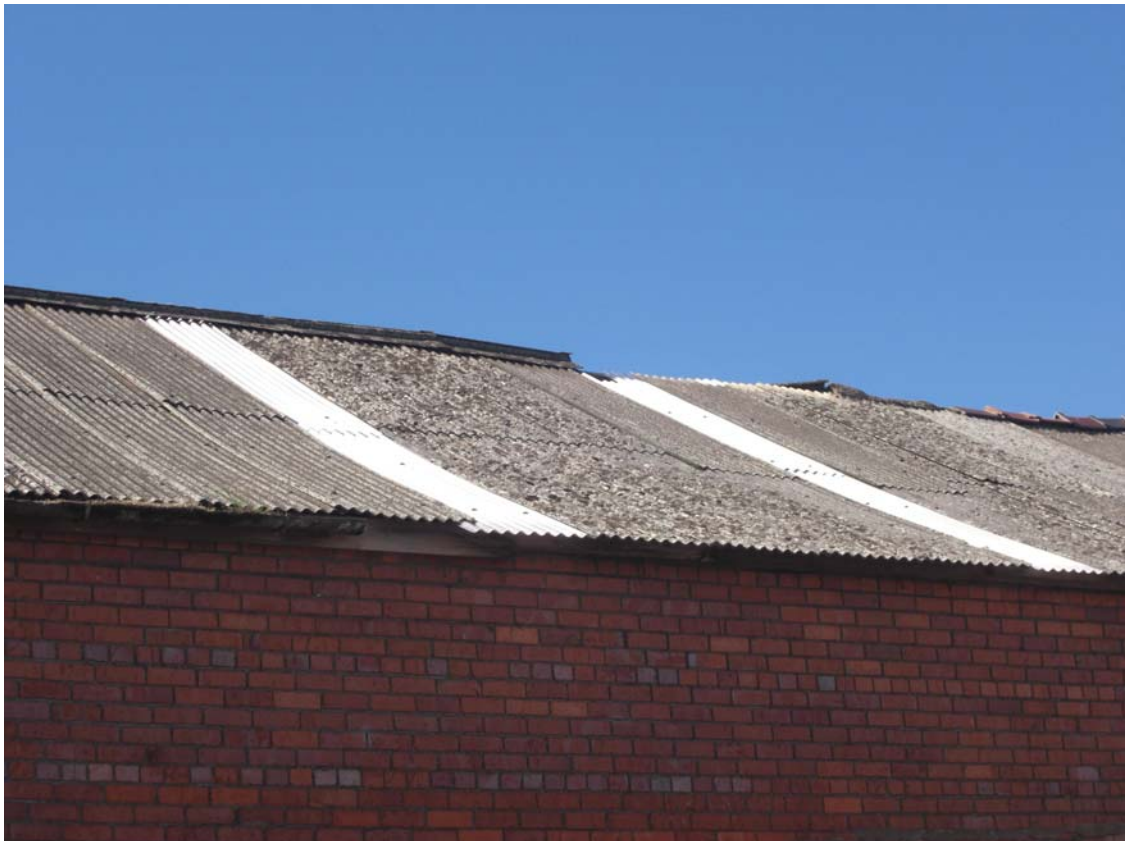
Missing Ridge Part B
