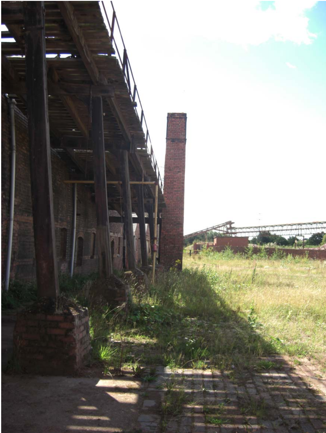
Rear of Part C Timber Runway Structure showing lean in support columns
