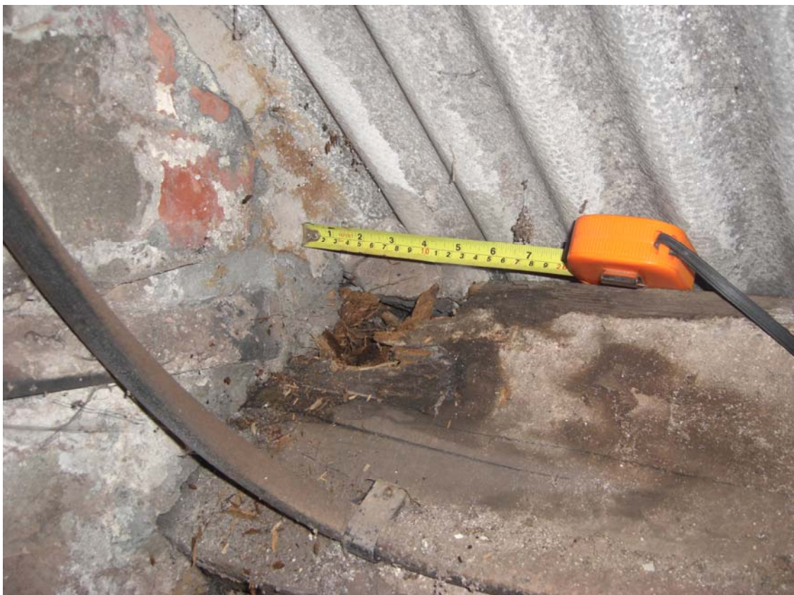
Trial detail examination of gutter support beam Part b showing extensive decay
