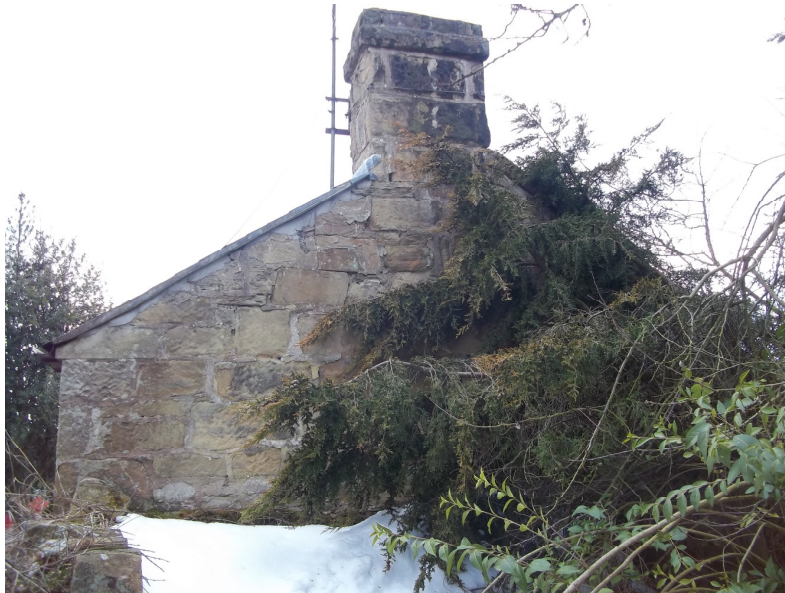
Picture 9 Side elevation (Vegetation against stonework)
