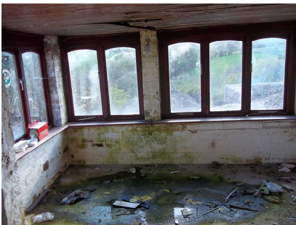
Picture 23 Disrepair of conservatory roof
