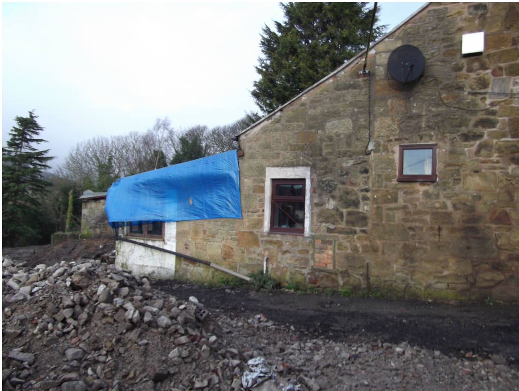
Picture 5 Side elevation indicating extent of extension with Vertical mortar joint.
