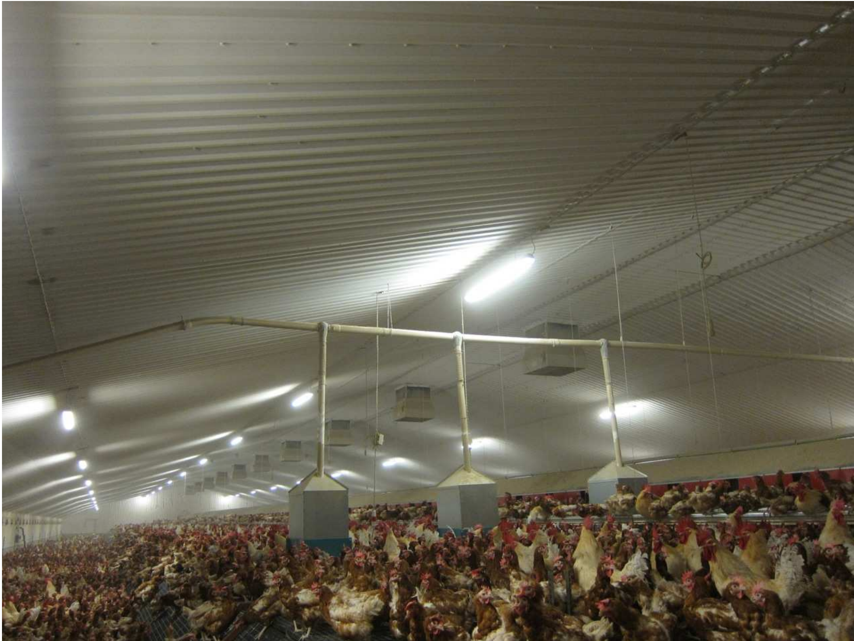
Ventilation fans are located at bottom of the vents on the roof.
