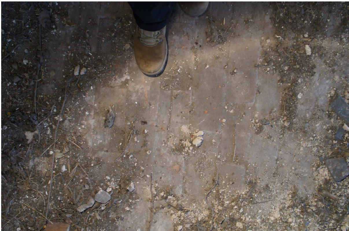
Figure 6: Bat droppings under central ridge
