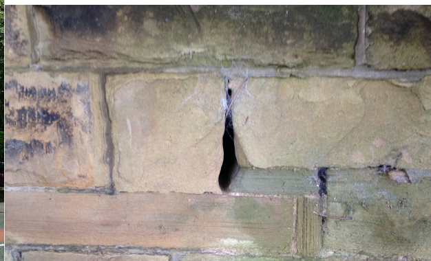
Photograph 2 showing one of the crevices in the stone work.
