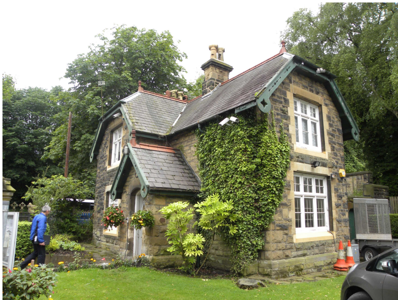
Photograph 4. Cemetery Lodge, showing roof and ivy coverage.
