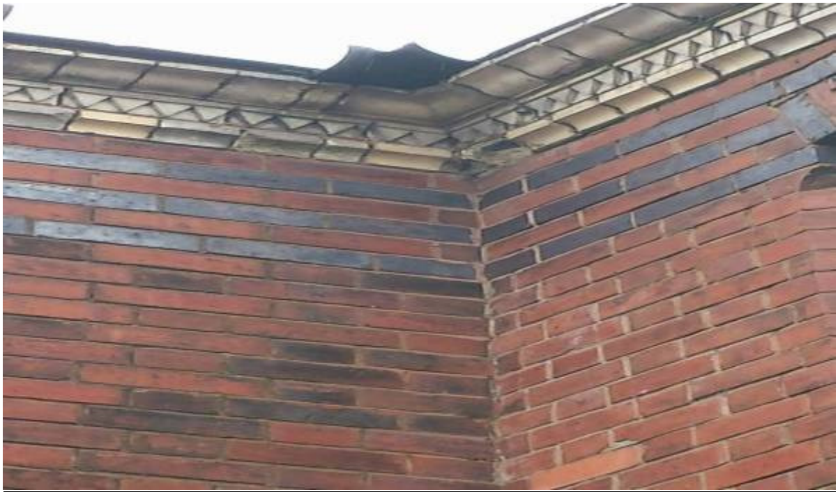
Absence of soffit boards on main house structure
