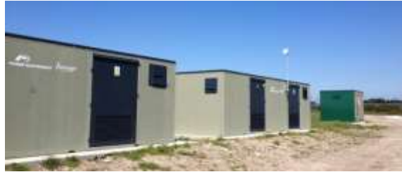
Inverter (centre), Little Trevease Solar Farm, Cornwall
