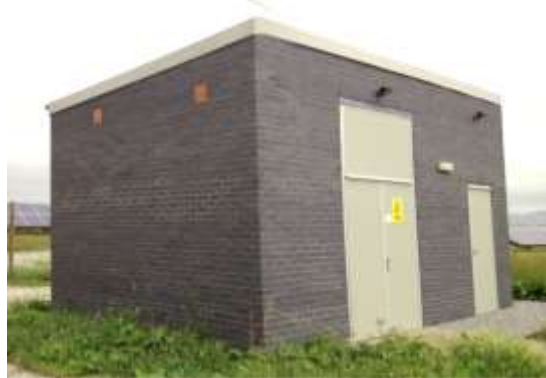
DNO Substation, Little Trevease Cornwall
