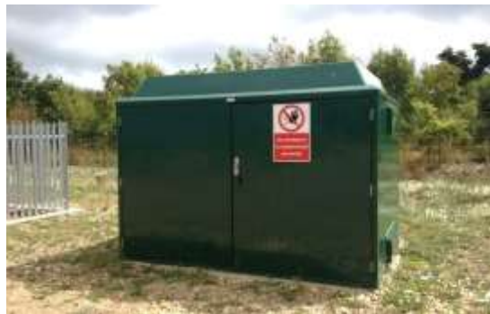
Customer Substation, Tavells Farm, Hampshire
