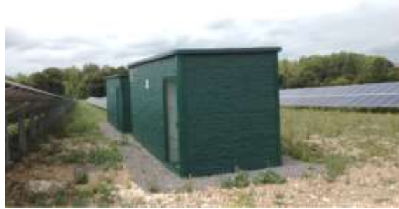
Inverter Building, Hatchlands Solar Farm, Devon
