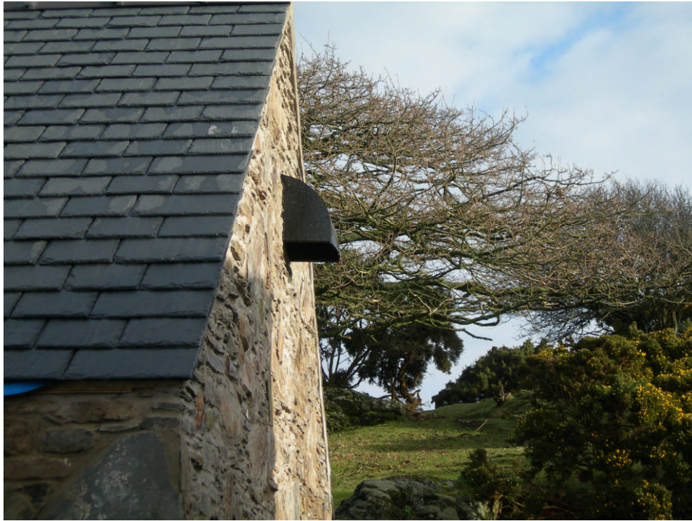
Above: Lesser horseshoe bat access cowling
