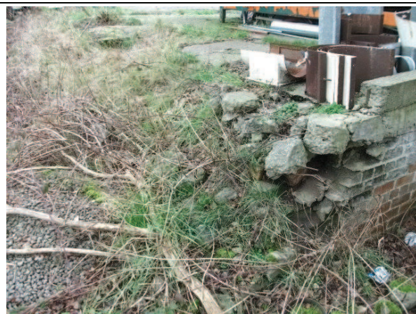
Photograph 7 – Rubble adjacent to hard standing area
