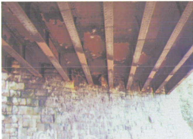
Plate 3- Underside of bridge B1 showing cavities.
