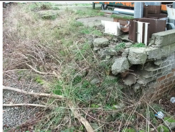
Photograph 7 – Rubble adjacent to hard standing area
