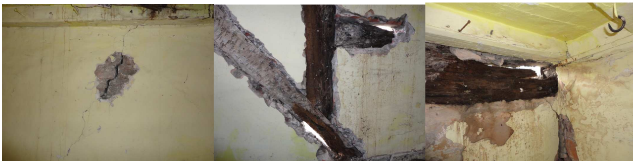
Photos showing the cracks in the timber framed (east) end gable wall as seen within the Store.
