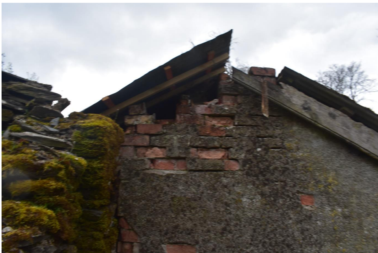
Figure 3.8: The damage to the rear gable wall of the kennels building.
