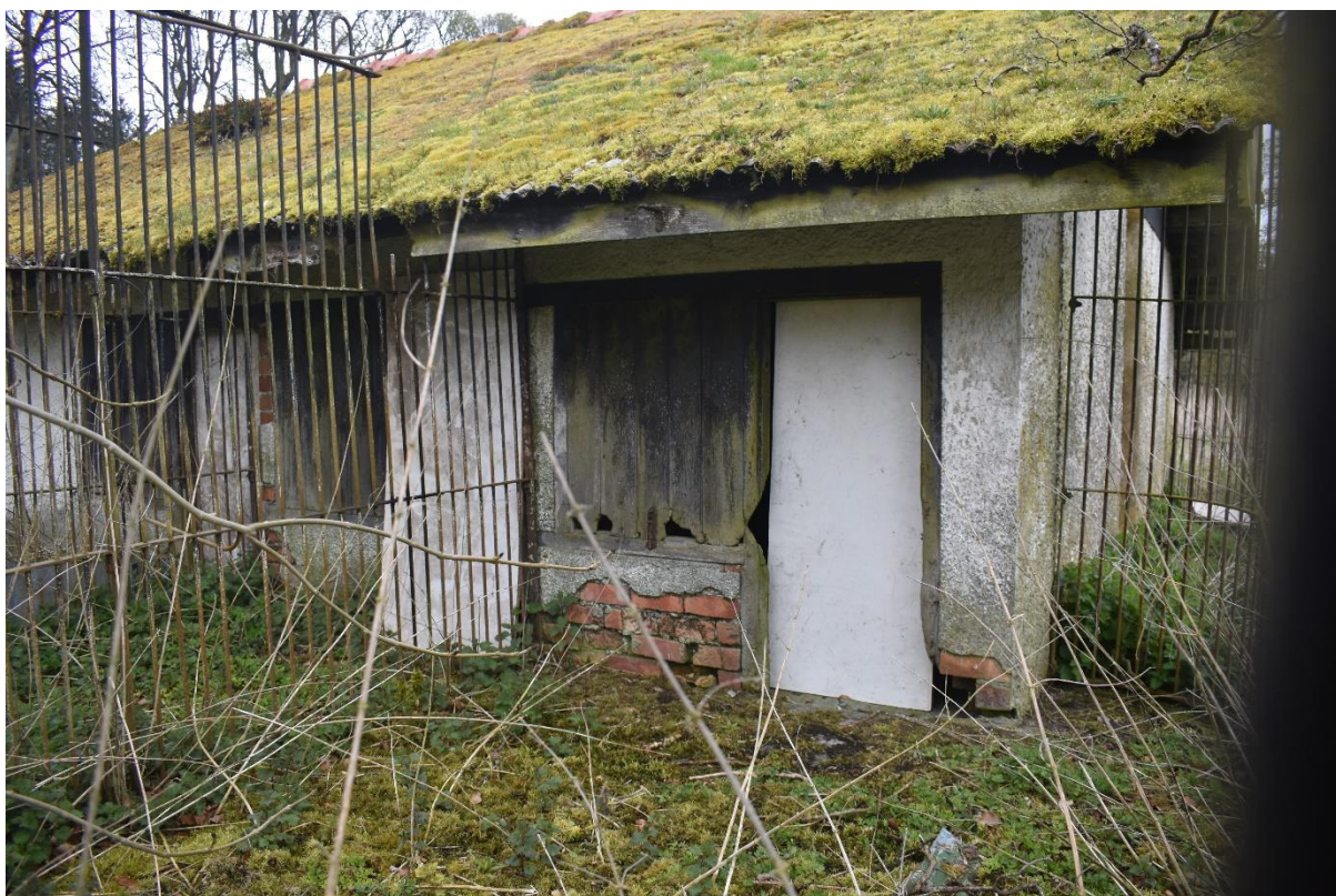
Figure 3.7: The points of access around the damaged doorways and windows.
