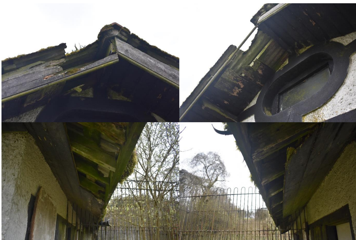
Figure 3.6: The damaged roofline of the kennels building.
