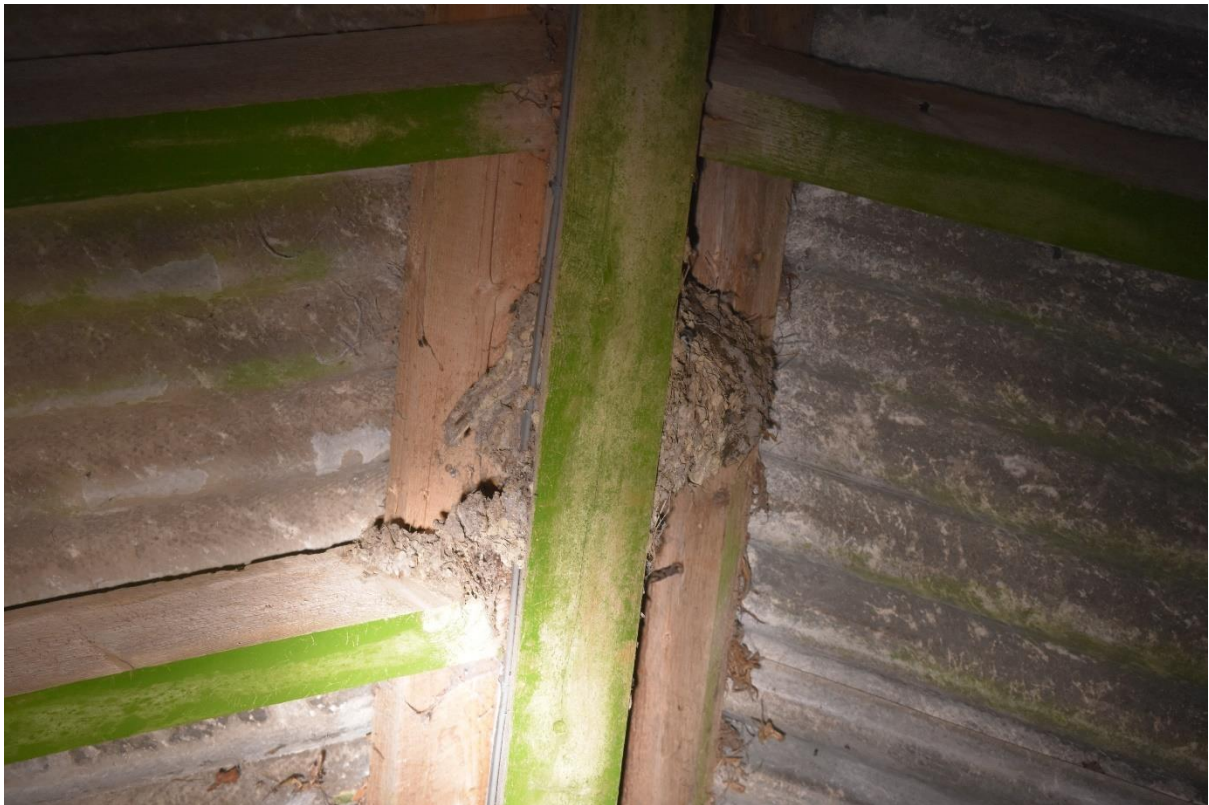
Figure 3.14: One of the swallow nests identified within the kennels building.
