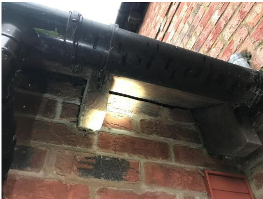
Plate 5 – A minor gap at the open eaves on the single-storey extension
