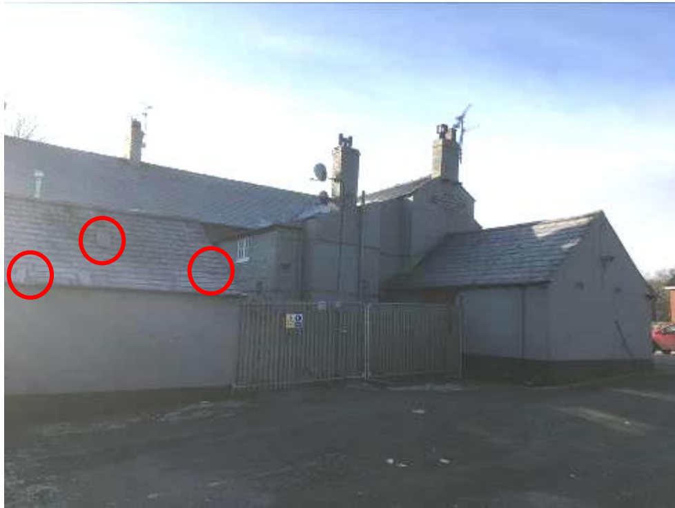
Plate 5: Northern elevations of B1 and B2 with missing/lifted slates on B2
