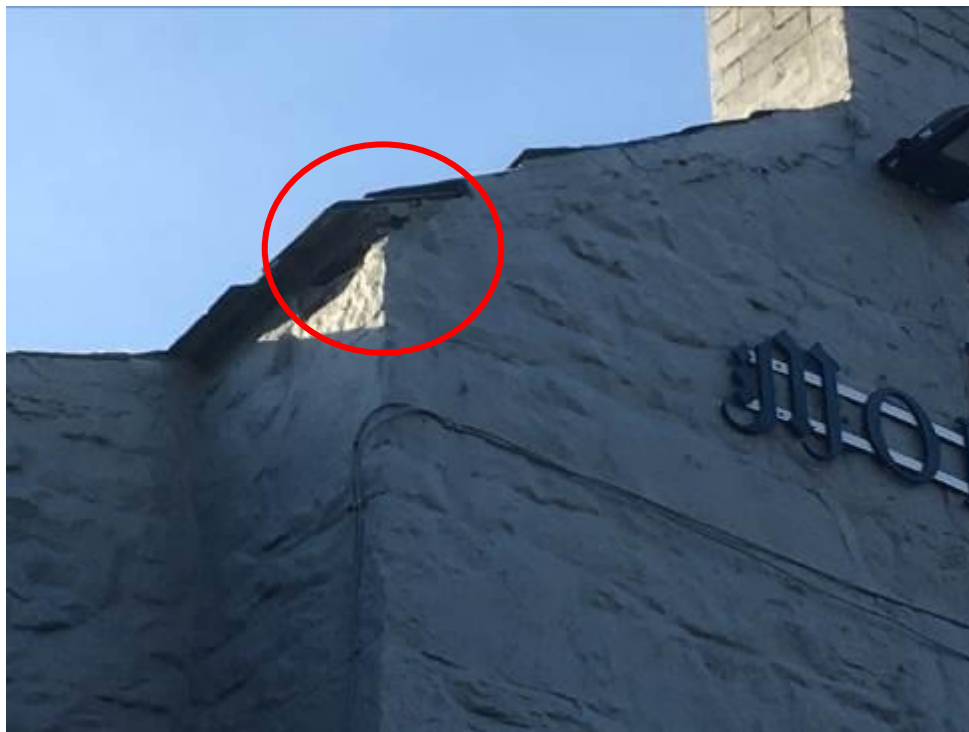
Plate 6: Gap at wall-plate level on the northern elevation of B1
