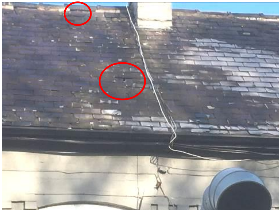
Plate 4: Gap between slates and under a lifted ridge tile on the southern elevation of B1
