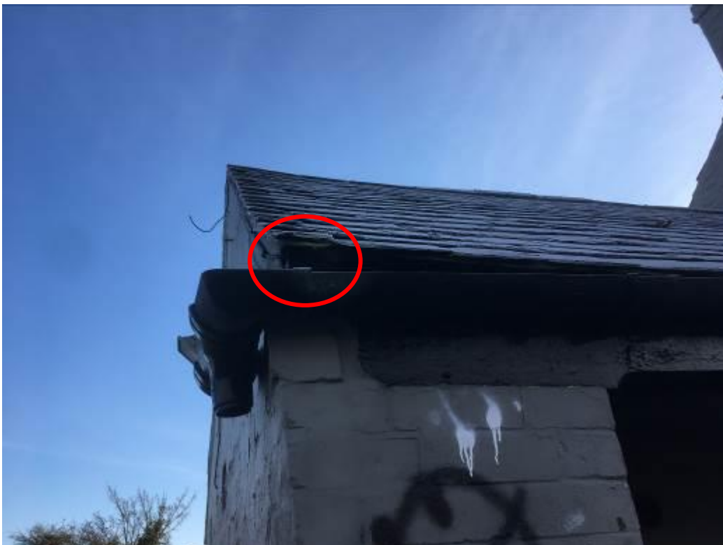
Plate 2: Gap beneath slates on the north-west corner of B1
