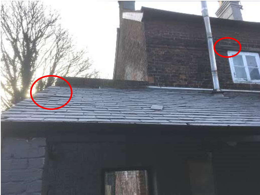
Plate 9: Northern elevation of B1 with lifted slates and window lintel crevice
