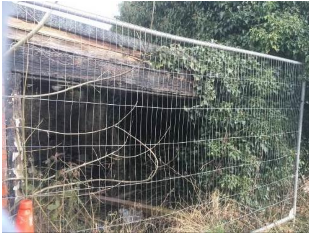
Plate 17: Derelict/collapsed outbuilding (Target Note 2)
