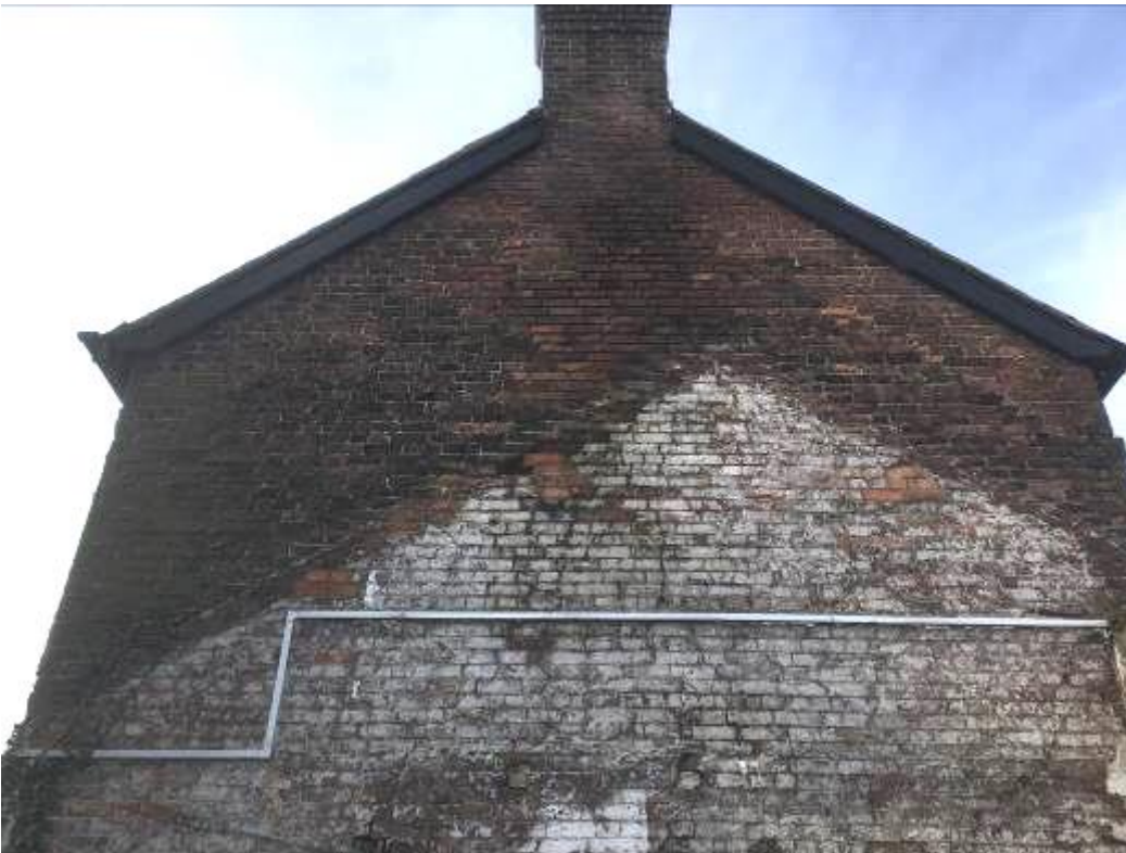
Plate 8: Eastern elevation of B1 with cracks in brickwork
