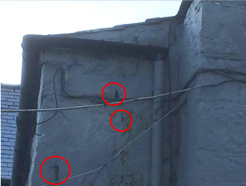
Plate 7: Gaps in the brickwork of the northern elevation of B1
