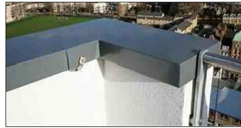
Typical Aluminum Capping Colour
