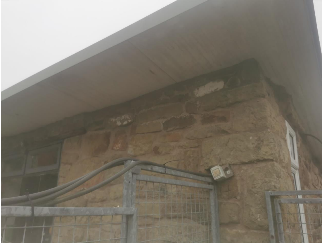
Photograph 3- Lack of gaps under roofing
