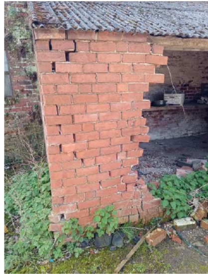
Photo 10 – Cracked and dislodged brickwork adjacent to opening.
