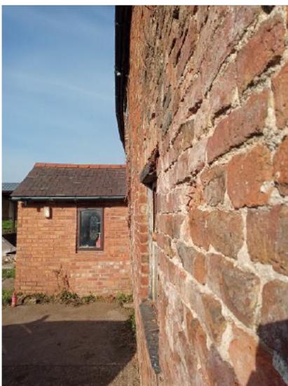
Photo 3 – Outwards bulge to front elevation.
