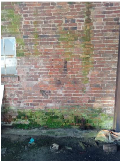
Photo 9 – Staining to elevation.
