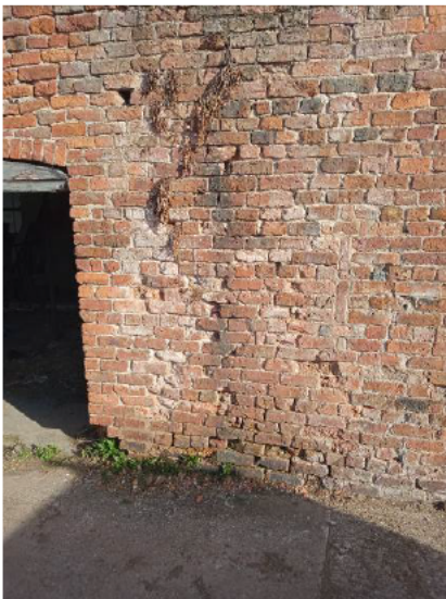
Photo 2 – Eroded brickwork and pointing.
