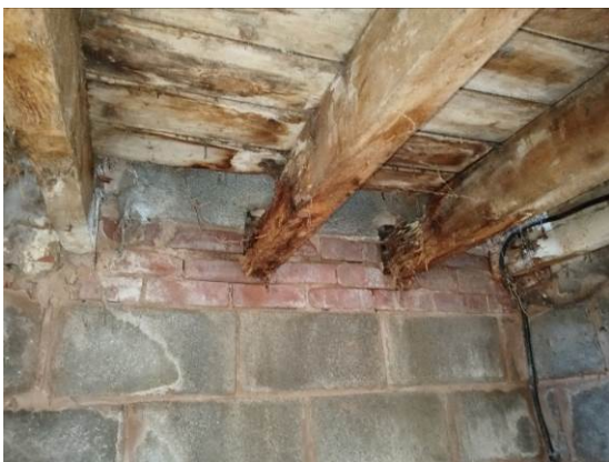
Photo 15 – Severe rot to floor joists.
