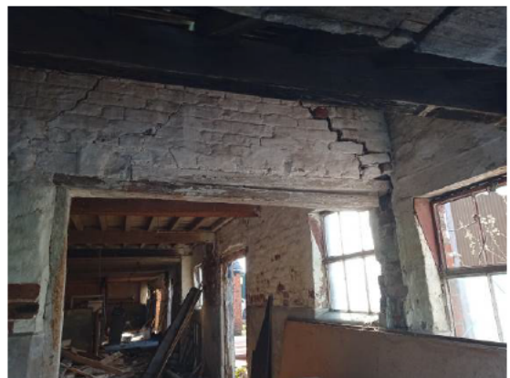
Photo 12 – Cracking to brickwork due to support removal from lintel.
