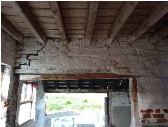
Photo 13 – Cracking to brickwork due to support removal from lintel.
