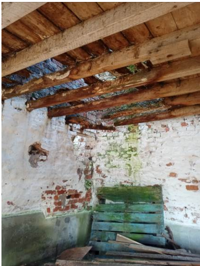
Photo 14 – Severe rot to floor joists.
