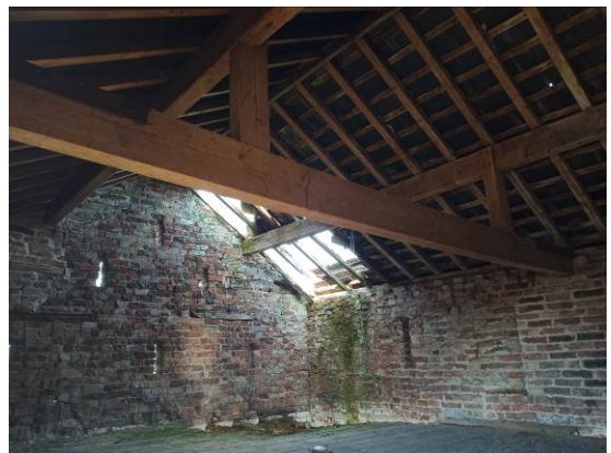
Photo 18 – Severe rot to roof timbers and staining wall walls..
