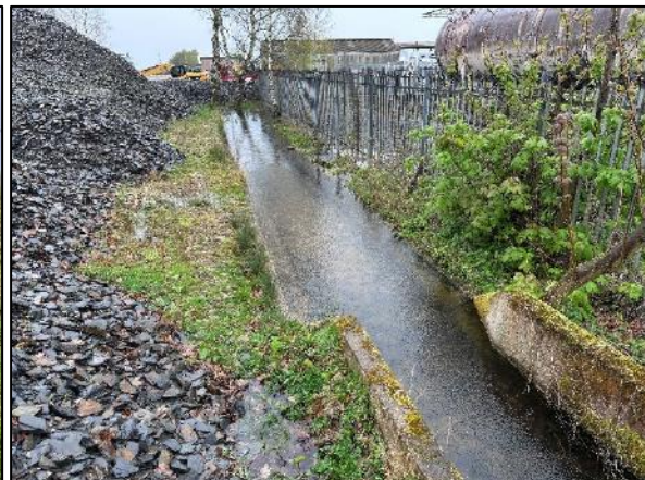
Figure 9: A flooded drainage channel (T1).
